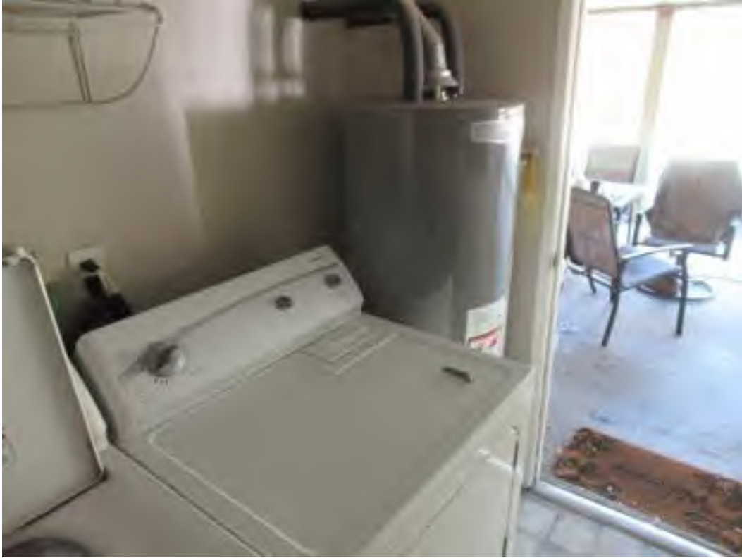
93. Gas-fired water heater at 18602 Altrudy Lane.
