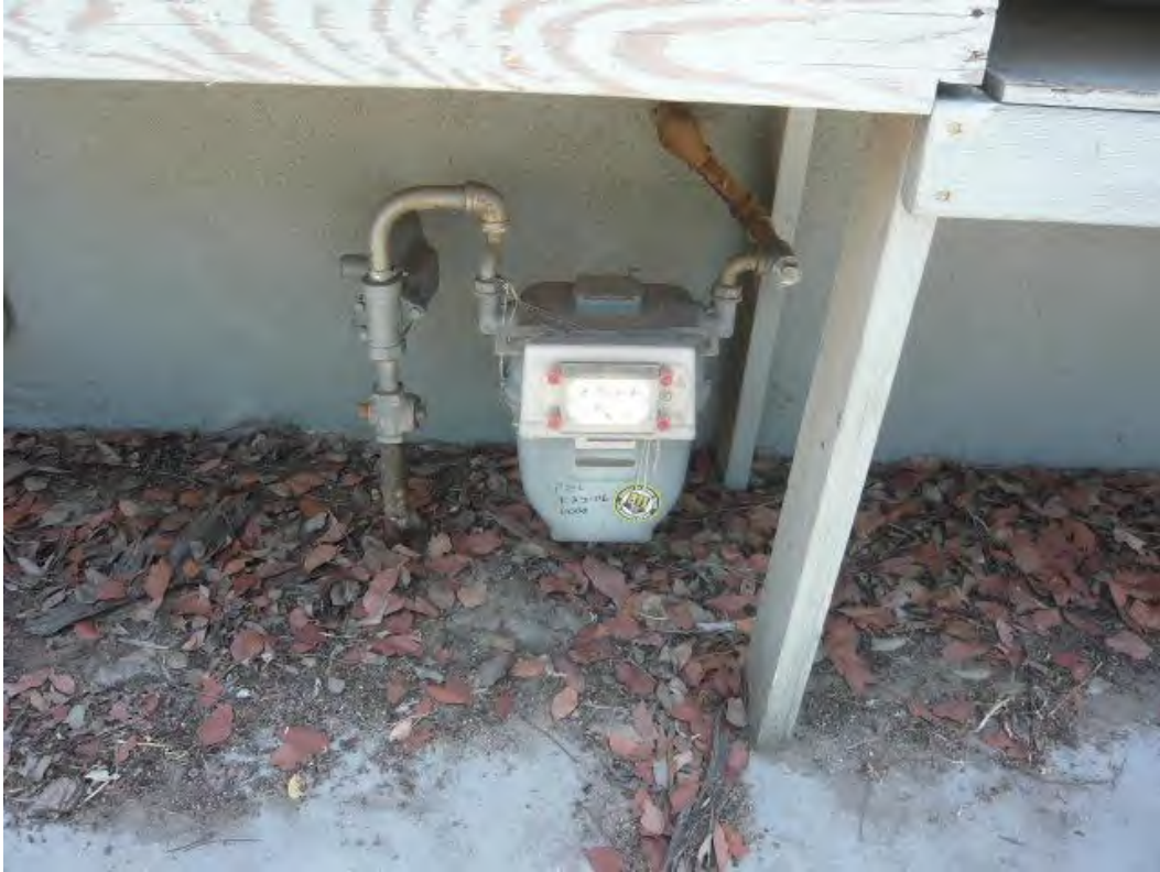
13. Gas meter at 18597 Altrudy Lane.
