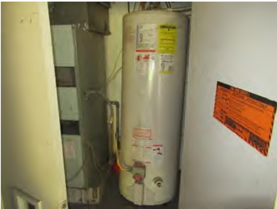
50. Gas-fired water heater at 18597 Altrudy Lane.
