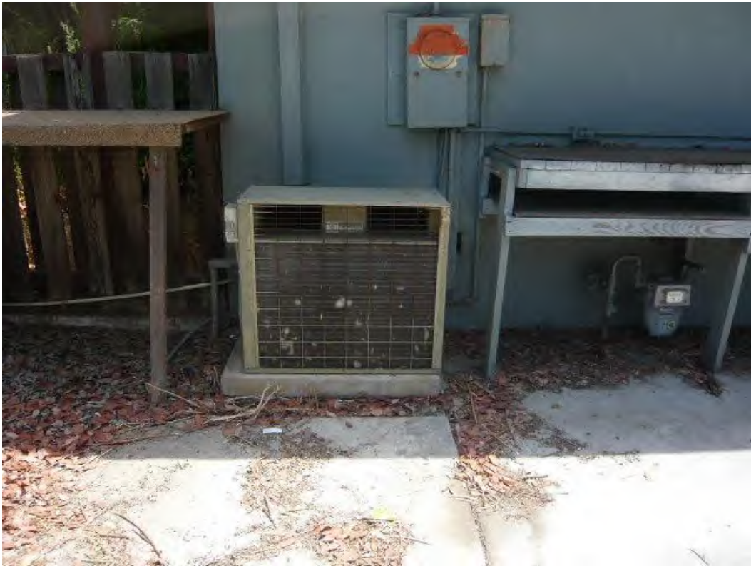
14. Pad-mounted condenser at 18597 Altrudy Lane.
