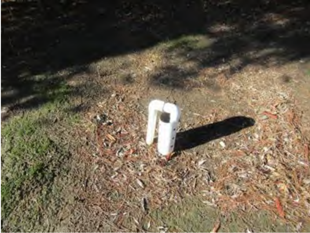
69. Pool overflow at 18602 Altrudy Lane.
