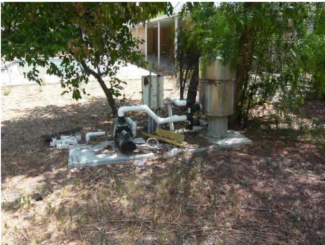
22. Pool filter provided at 18602 Altrudy Lane.
