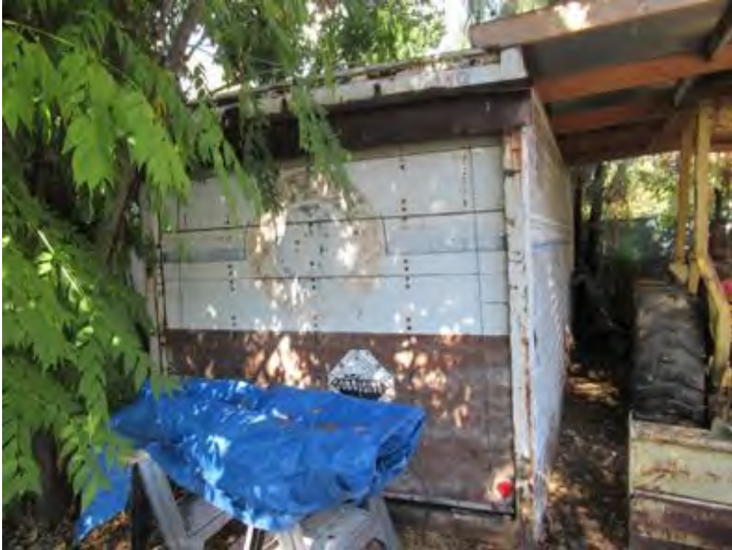
21. Storage container at the north side of the subject property at 18597 Altrudy Lane.
