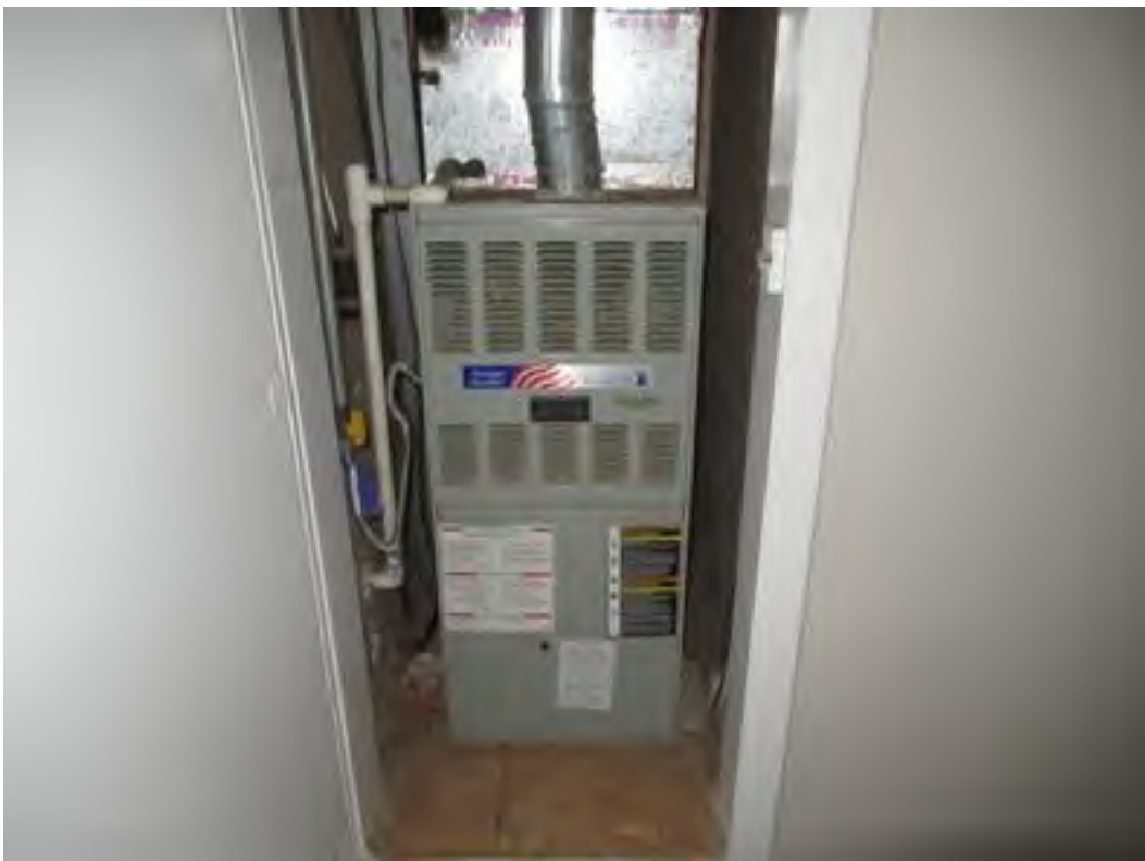
94. Gas-fired forced air unit at 18602 Altrudy Lane.
