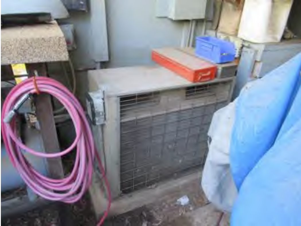
49. Pad-mounted condenser at 18597 Altrudy Lane.
