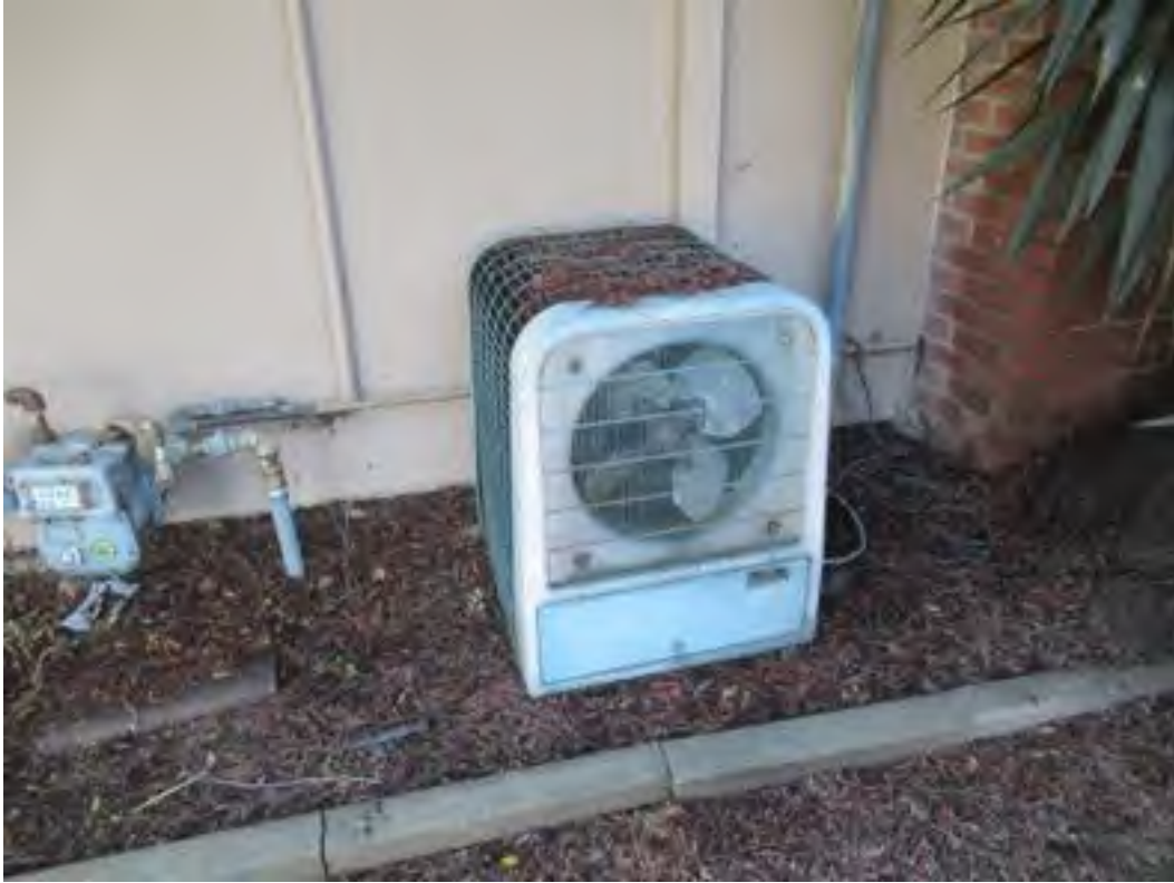
95. Pad-mounted condenser at 18602 Altrudy Lane.
