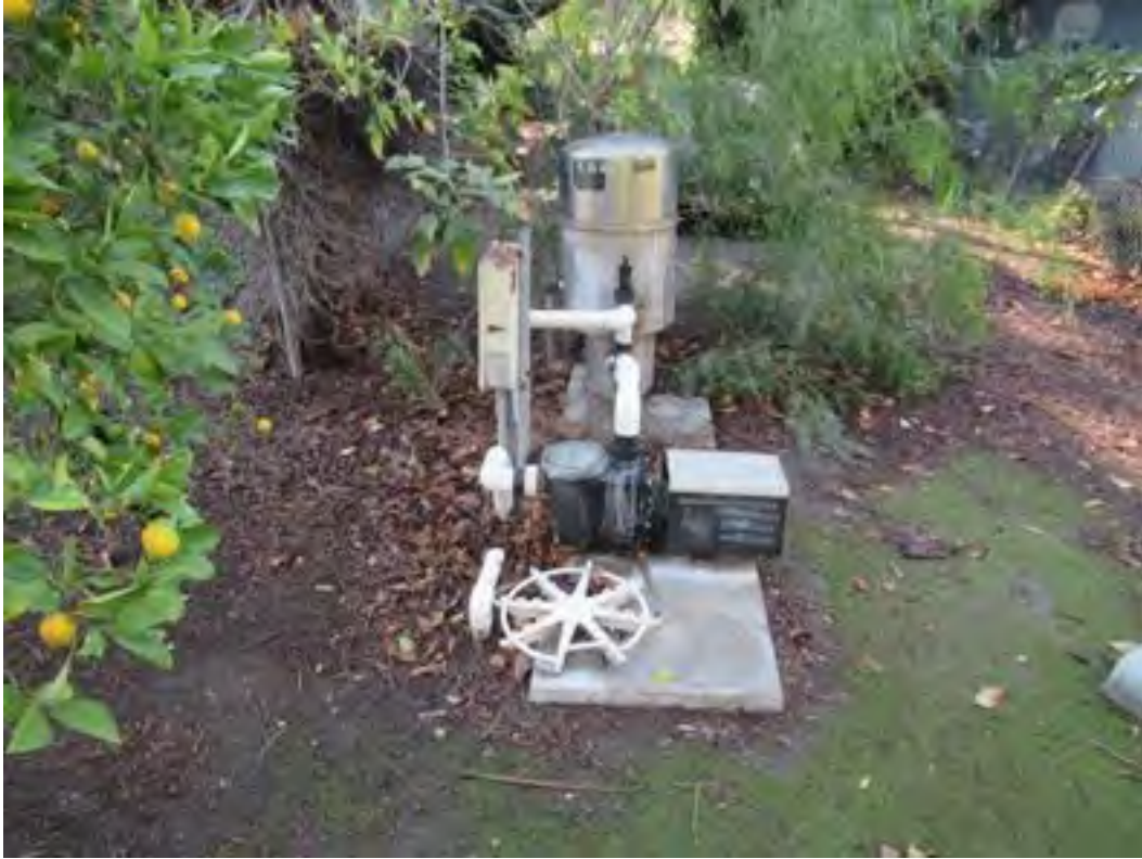
67. Pool filter provided at 18602 Altrudy Lane.
