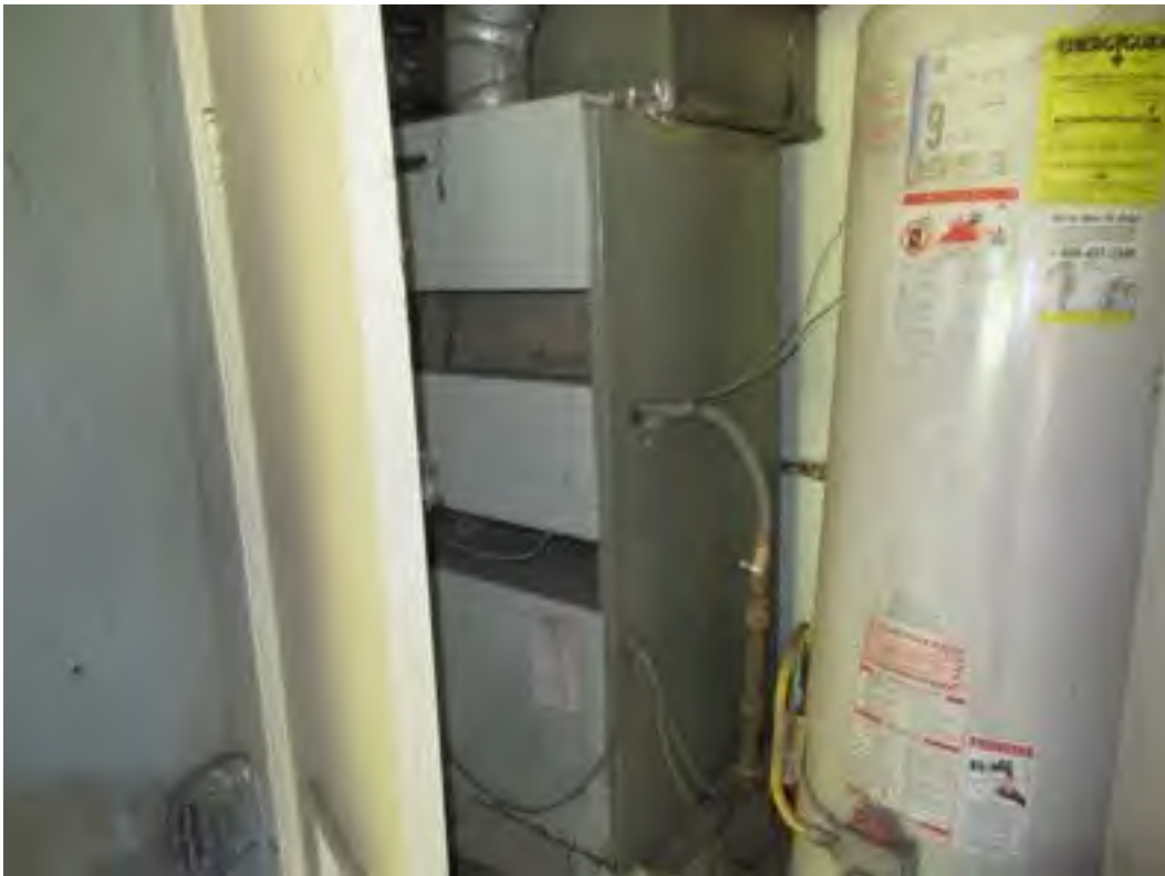
48. Gas-fired forced air unit at 18597 Altrudy Lane.
