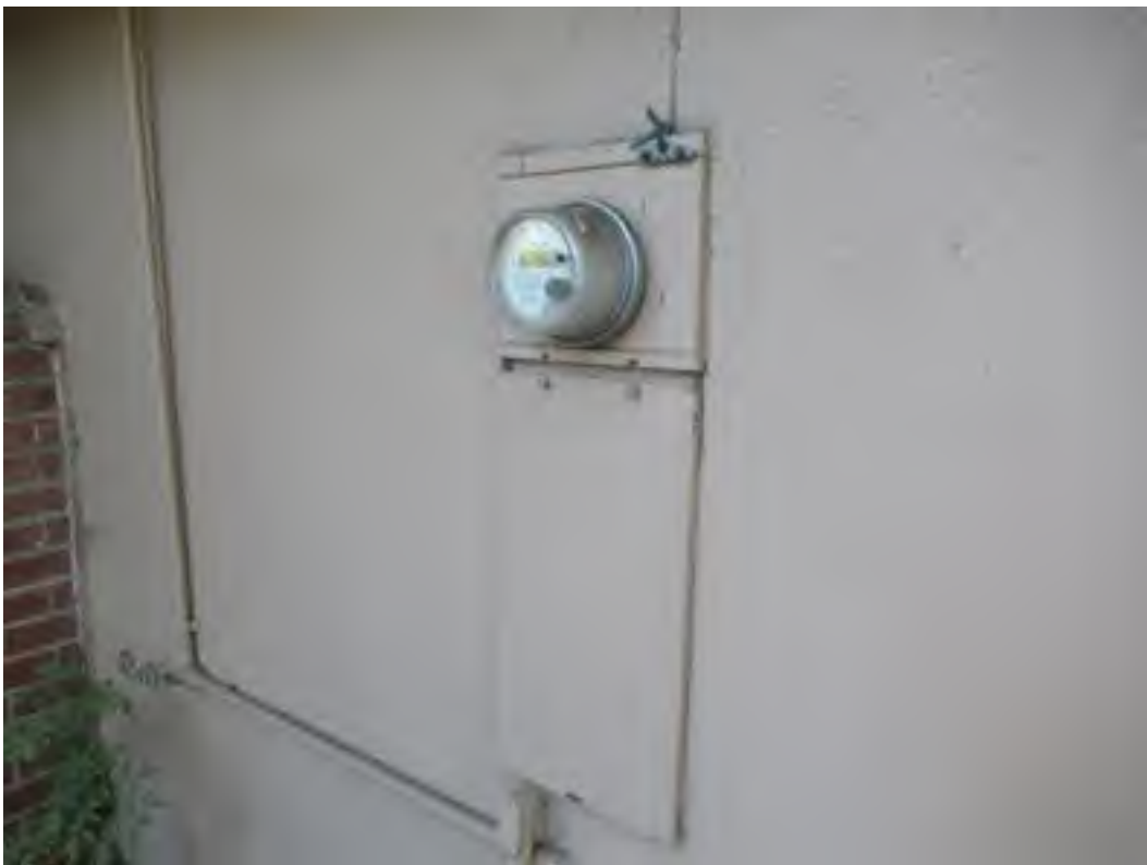
92. Electric meter at 18602 Altrudy Lane.
