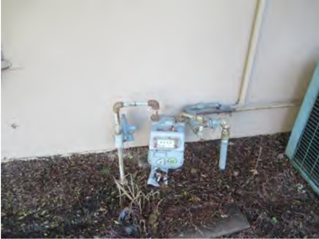
91. Gas meter at 18602 Altrudy Lane.
