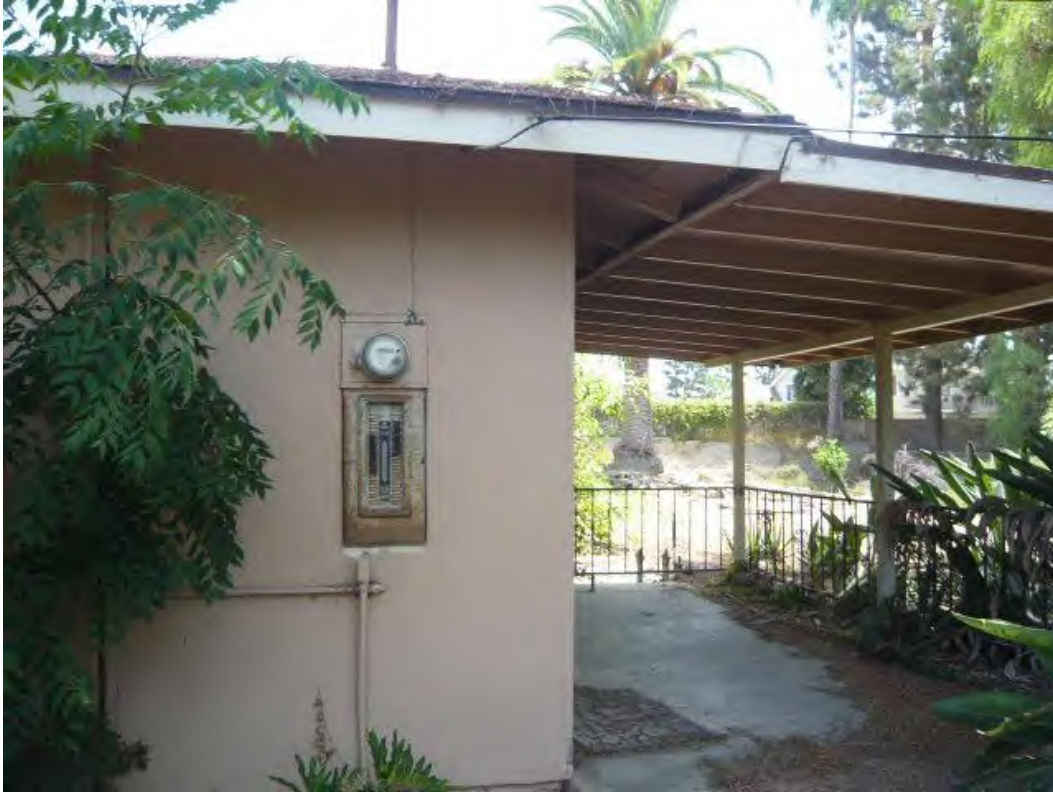
33. Electric meter at 18602 Altrudy Lane.
