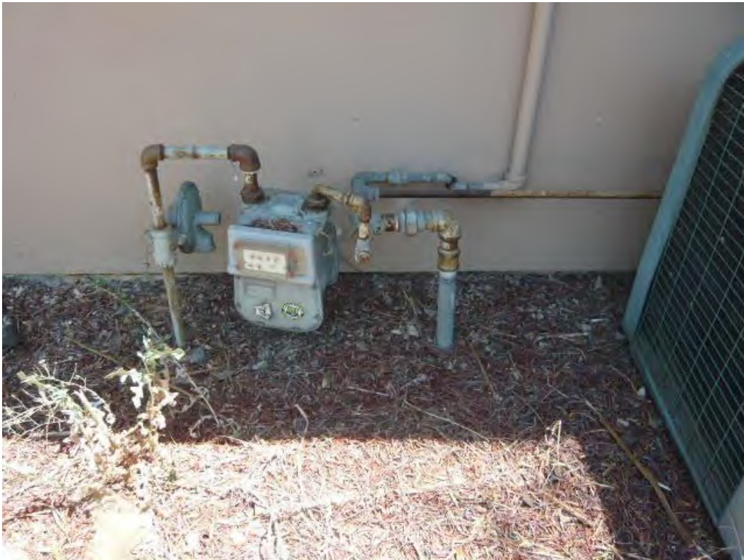
32. Gas meter at 18602 Altrudy Lane.
