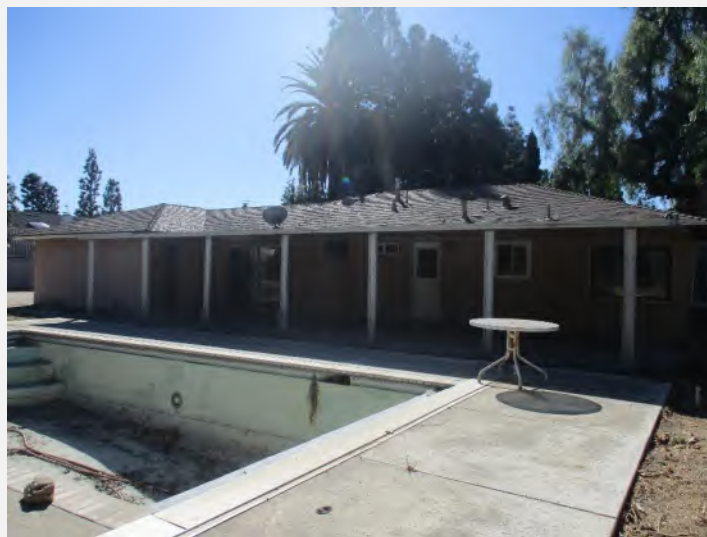
Photograph 2. Rear (north) elevation of the residence at 18602 Altrudy Lane, view looking southeast. Photograph taken on October 22, 2024.
